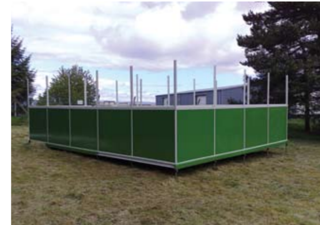
6 The shelter with all of the lower sections of the wall panels in place and the cruciform in place for the upper wall panels and window sections.
