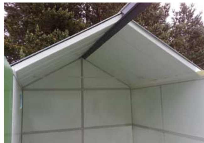
9 A cross-section view of the roof showing the lightweight GRP and foam core panels which provide the high levels of insulation.
