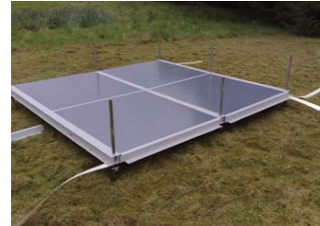
2 Once the floor beams are all in position the insulated floor panels are slid into place between the beams.
